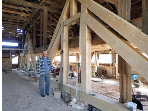
Master timber framer Steve Fifield of Canterbury with the trusses designed by Fire Tower Engineered Timber that support the roof of the new Carriage Barn.
